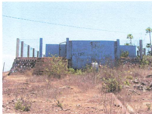
Gambar 4.6. Reservoir Ground TVRI Kapasitas Tampung 400 m 3 (Dokumentasi, 2011)
