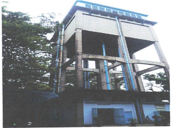
Tangki Reservoir Kuwak I
