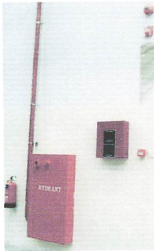
Gambar 6.15 Indoor hydrant box
