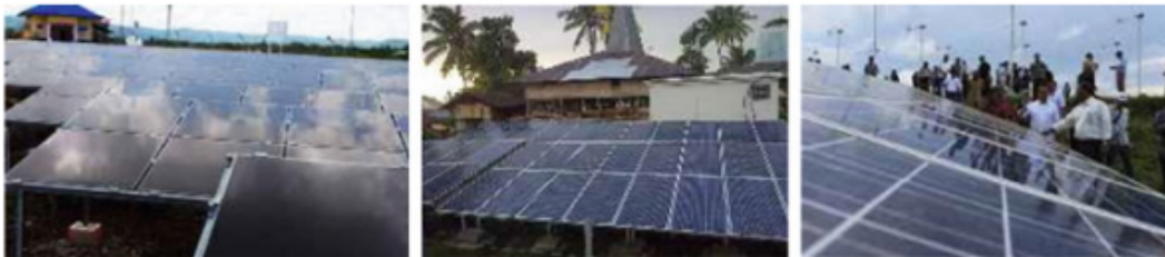
Fig. 19.7 Installed solar panel system
