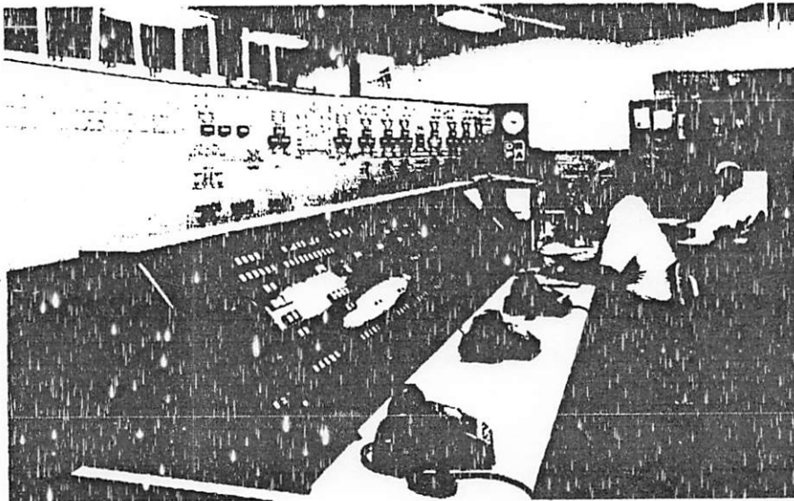
FIGURE 17.—Central Train Control Facility
