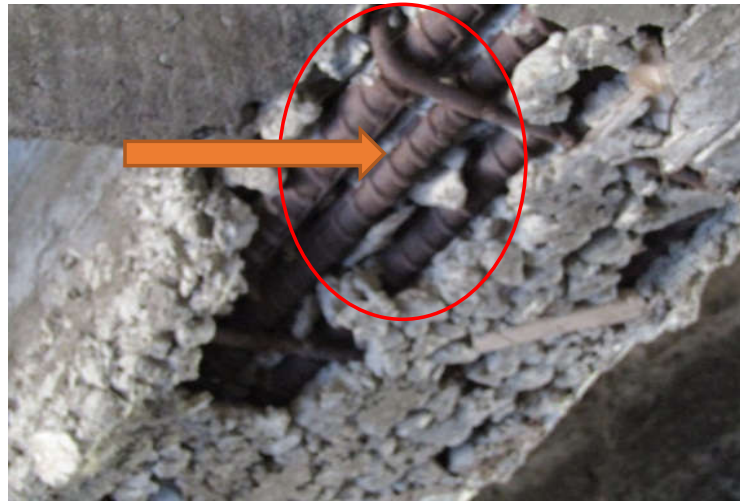
7 GELAGAR BETON KEROPOS
