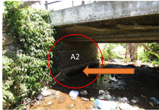
ABUTMENT TERKIKIS (A2)
