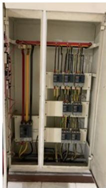
Gambar 1 Panel Main Distribution Panel
