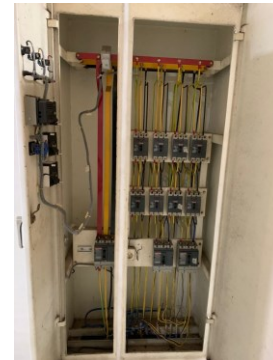
Gambar 2 Panel Sub Distribution Panel
