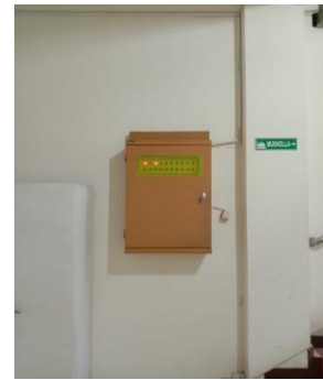
Gambar 14. Panel Lampu Penerangan Laboratorium EBT
