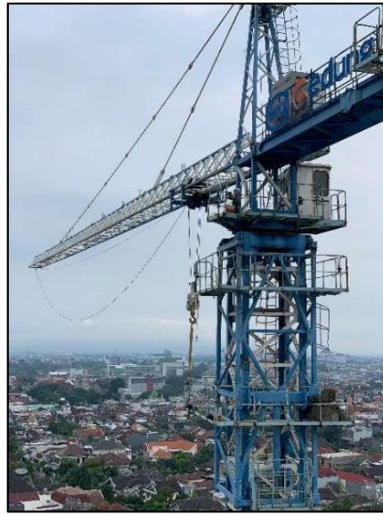
Gambar 4. 5 Tower Crane 6520/10 E nomor seri 1012TC1700650
