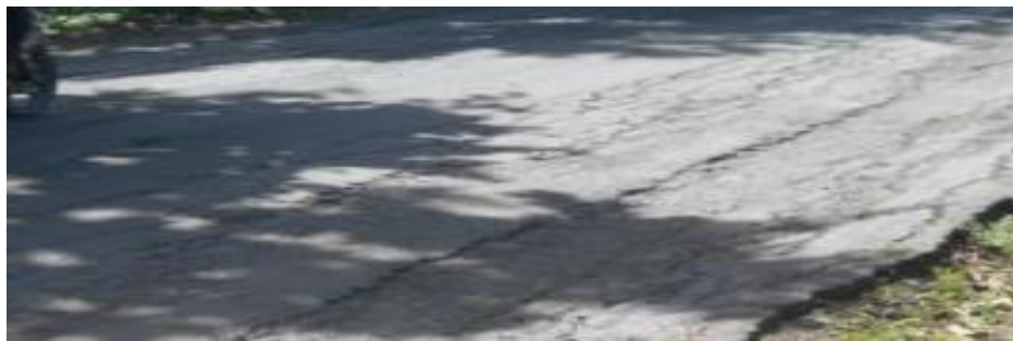
Gambar 2. 14 Kerusakan Retak Turun ( Crack With Depression )
