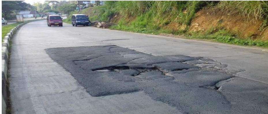
Gambar 2. 9 Kerusakan Tambalan ( Patching )
