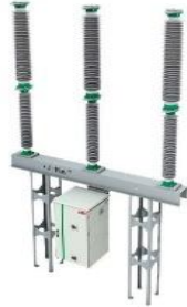
Gambar 2. Circuit Breaker (CB)
