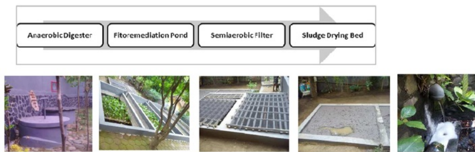
Figure 4. Condition Processing Unit WWTP Tlogomas
