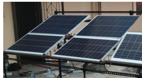
Figure 3.12 Solar Cell Panel
