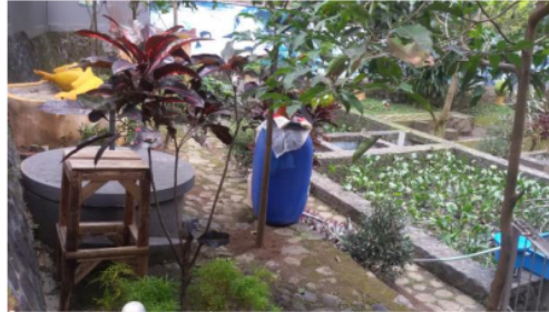
Figure 1. The Condition of IPAL Communal Tlogomas, Malang (2017)
