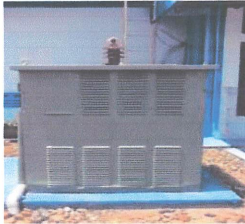
Gambar 2.4 Neutral Grounding Resistance
