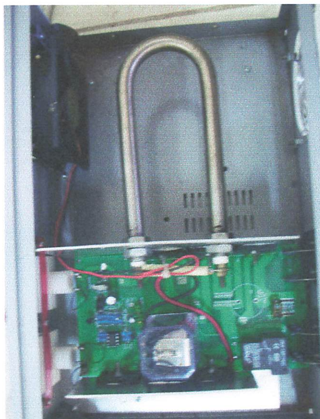
Gambar 4.30 Automatic Win Generator Charger Control
