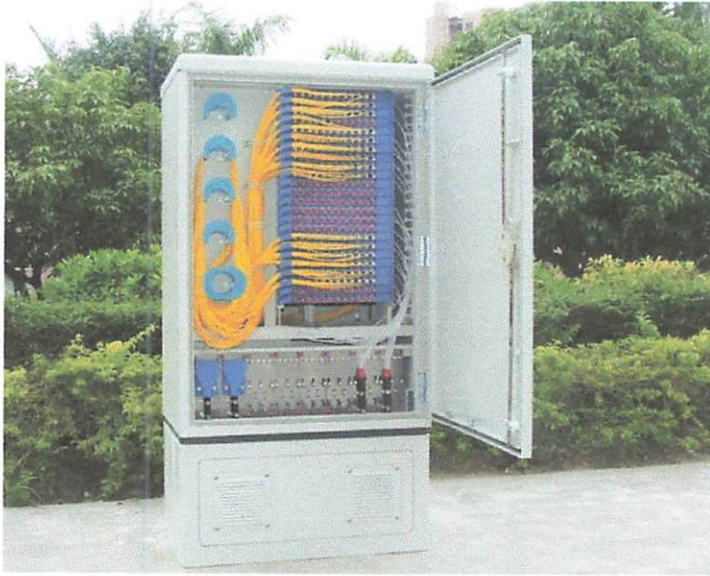
Gambar 2.8. ODC ( Optical Distribution Cabinet ). [3]
