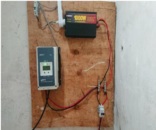
Gambar 4.5 Instalasi solar home system.
