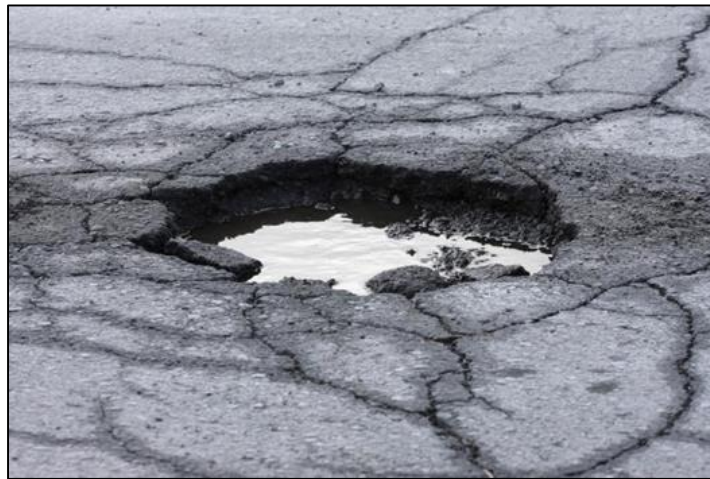
Gambar 2. 3 Lubang ( Potholesi ) (Bina Marga, 2011)
